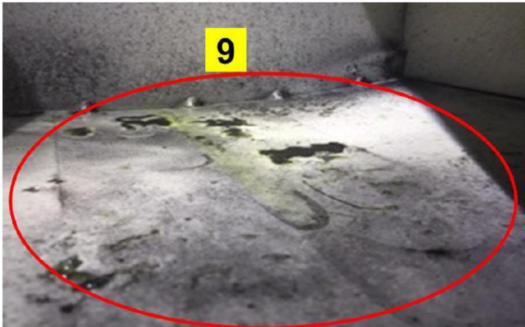
9. Oil and debris identified in back corners of gantry
