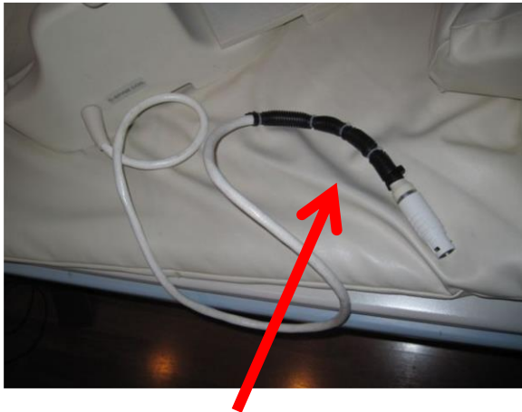
Coil with plastic tubing and zip ties used to cover damaged cable
